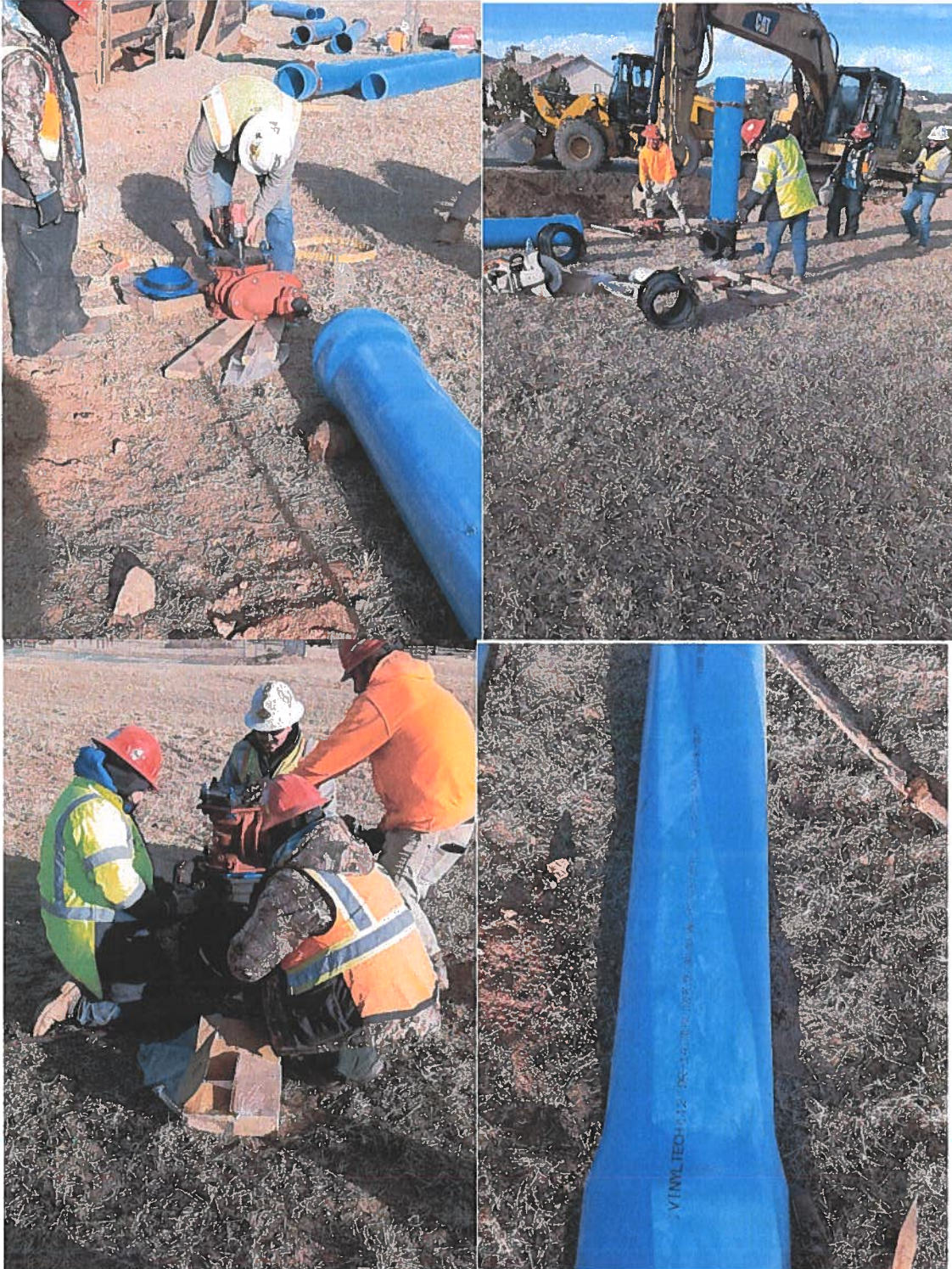
Assmbling the 12"x8" T, Foster adapter, 8" Gate Valve and 12" DR-14 C100 PVC Pipe:
